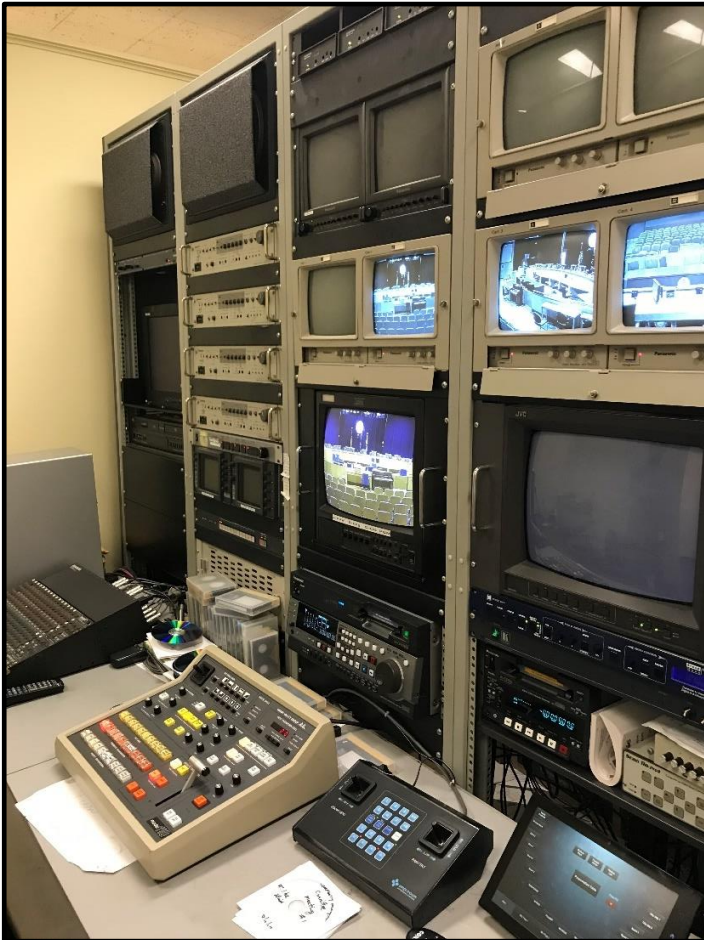
Figure 3: Existing Video Equipment and Controls
