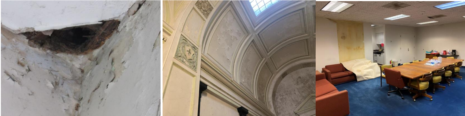
Photos from left: NOPD building with termite damage, Orleans Parish Criminal District Court's Grand Hall deterioration, and water damage within jury deliberation rooms
