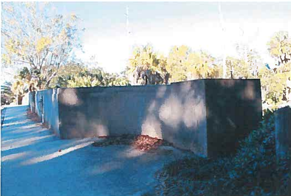
Condition Photo 3: Debris accumulation on sidewalk (northeast corner of Recall No. 102226 shown).
