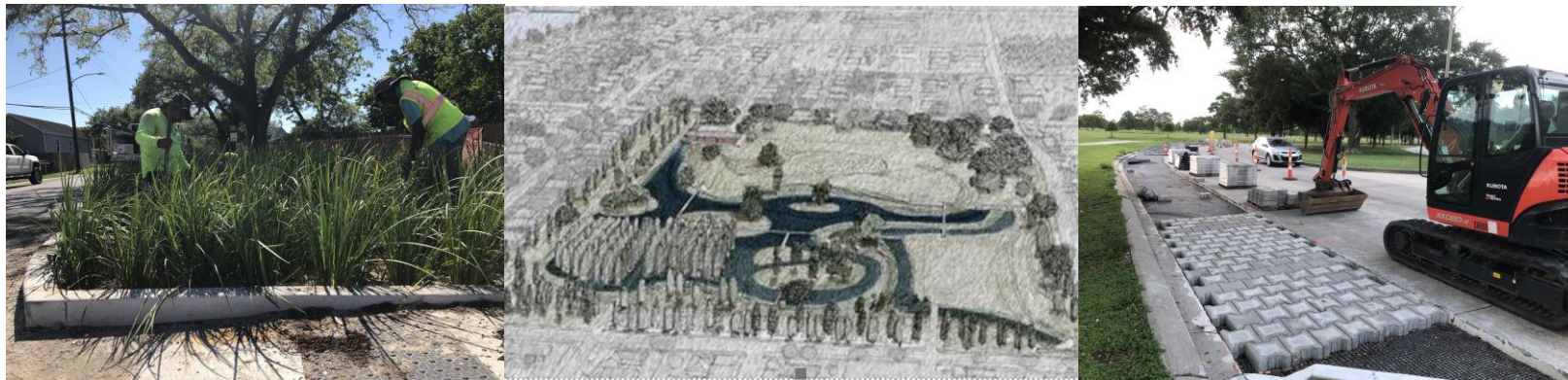
Photos from left: DPW Rain Garden, Mirabeau Gardens, DPW Permeable Off-Street Parking Pavers Source: Staff Photos and Resilience Renderings
