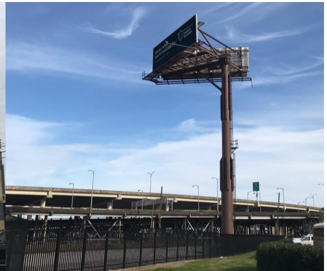
Figure 12. Example of billboards in V-type configuration with monopole support structure.
