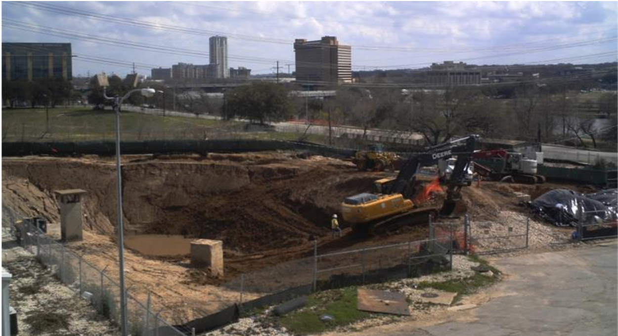
Figure 6. Photo of Seaholm cleanup. http://kut.org/post/seaholm-substation-cleanup-complete
