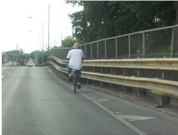
St. Claude Bridge poses major hazard for cyclists
