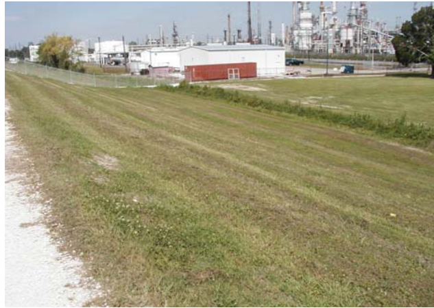
Picture from top of levee (future paved bike path) downriver of Murphy Oil in St. Bernard Parish
