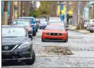
A driver sizes up a pothole on Felicite Street before driving around it Wednesday.
