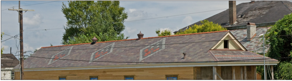
This distinctive slate roof with diamond patterns, terra cotta ridge caps, and Chinese caps are being retained as part of the rehabilitation project.
