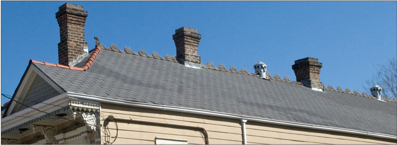
Ridge caps are located along the roof hips, cresting is along the top ridge and a finial is found at the end of the main roof gable. Chimney placement reflects the internal organization of the residence and Chinese caps provide roof ventilation.
