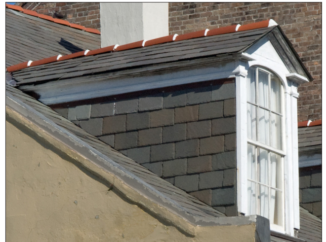
This gable roof dormer is appropriately located, proportioned and detailed for the building and include slate cheek walls. Spanish tile ridge caps should be retained.
