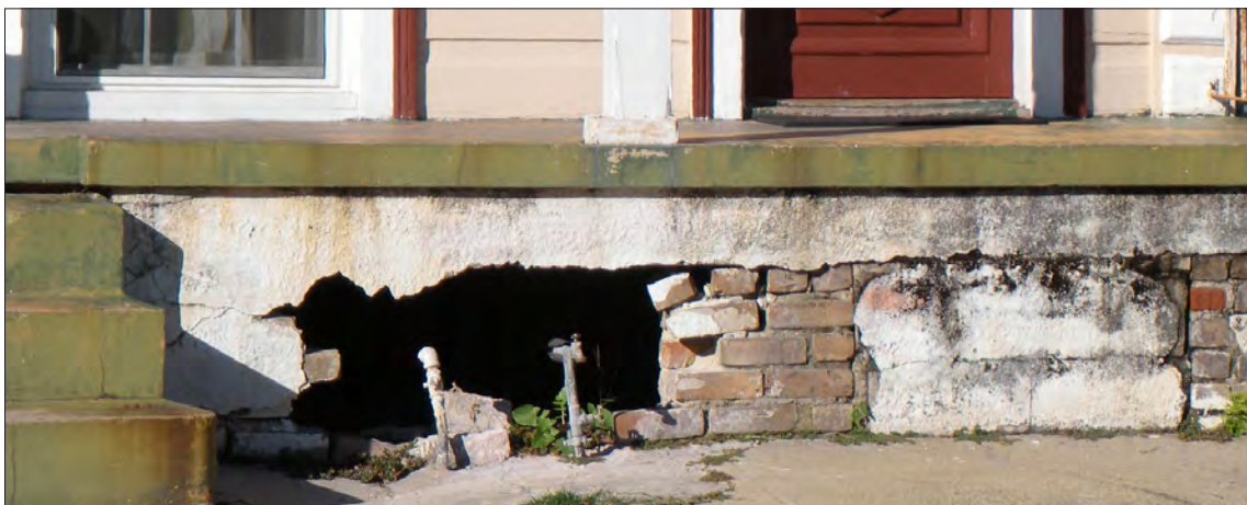
The stucco plaster has not been maintained and the bricks under the porch post are collapsing. The dislodged bricks can lead to structural problems at the porch if not repaired.
