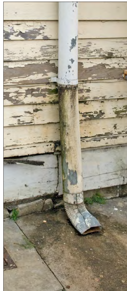
The downspout is discharging immediately adjacent to the building onto a concrete surface. The bottom of the downspout is crushed, likely resulting in clogging. The storm water splashing onto the concrete surface can saturate the wood wall and masonry foundation. The wood adjacent to the downspout is bare with visible deterioration.
