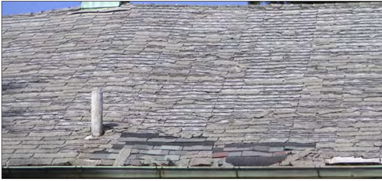
The mineral granules on the asphalt shingles have almost completely worn away. Portions of shingles have broken off and can be found in the gutters and on the ground. Prior patching is evident at the edge of the roof. The top of the roof curves down from the chimney, a possible indication of a structural problem.
