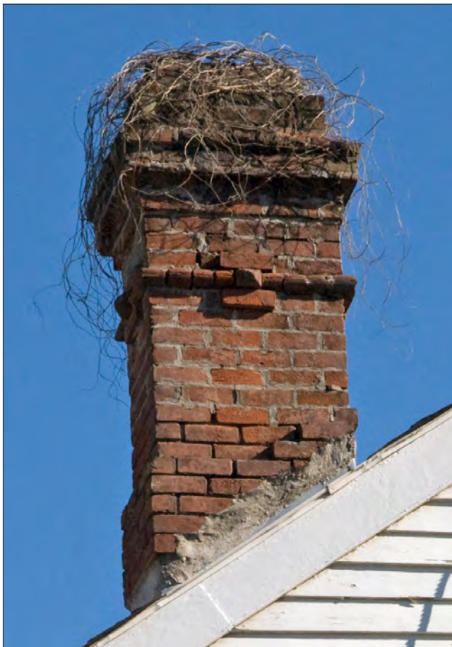
The chimney is leaning with several open joints visible. Rebuilding matching existing detailing is recommended.
