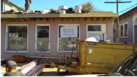
A building under renovation on Broad St. now houses a bicycle shop.
