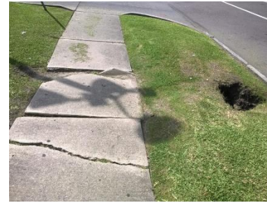
Sidewalk in need of repair
