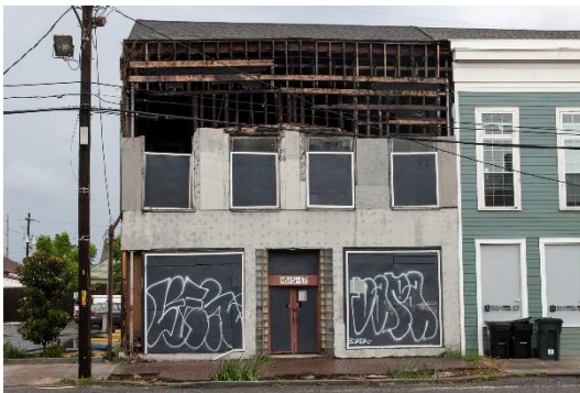
Re-investment is underway, yet remaining vacant buildings on the corridor are in need of substantial renovation.
