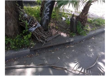
Storm drain in need of repair
