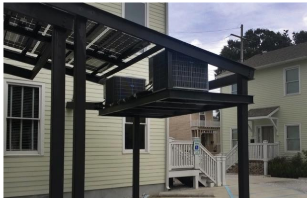
Elevated HVAC unit Elevating HVAC units high allows access underneath.
