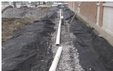
French Drain Installation A french drain is long, narrow, gravel-filled ditch that catches and treats stormwater runoff.
