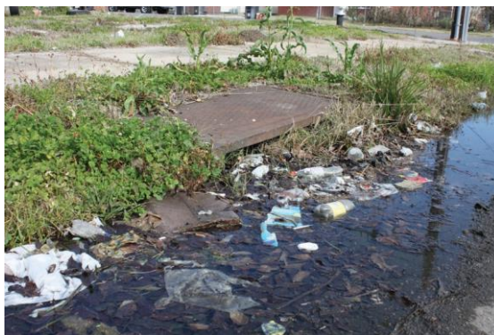
Clogged Catch Basin
