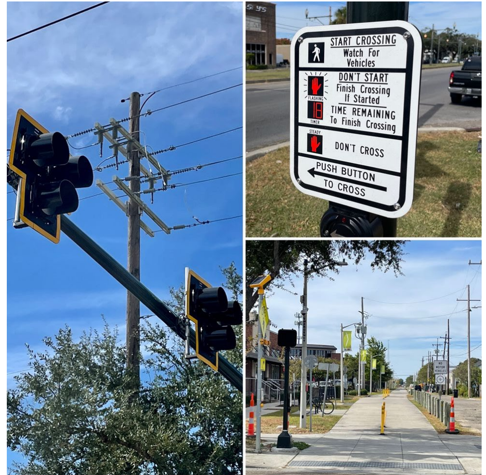
Pedestrian Hybrid Beacon installed at Lafitte Greenway and N. Carrollton Avenue
