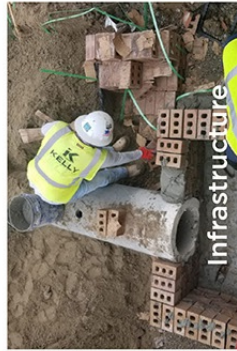
Infrastructure This includes the repair and replacement of drain lines, sewer lines, and other utilities.
