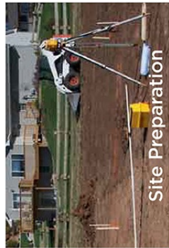
Site Preparation This includes protection of vegetation (including existing trees), erosion sediment control, clearing and demolition, and excavation.
