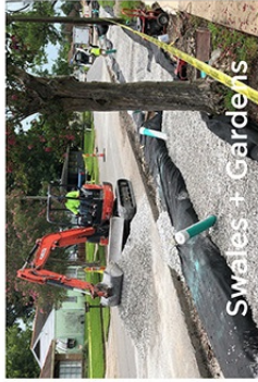
Swales + Gardens Installation of bioswales and rain gardens, including subsurface materials such as gravel, with plantings above. This includes the installation of a bioswale in the Pontchartrain Park neighborhood.
