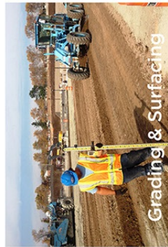
Grading & Surfacing This includes the shipping of earth to desired elevations. This includes backfilling any excavations that have been made, and then the placing and compaction of soils. This is followed by the installation of surfacing materials such as concrete for walking paths and basketball court.
