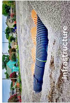
Infrastructure This includes the installation of drain lines, utilities, and stormwater storage systems (SWS) for stormwater at Easton Park.
