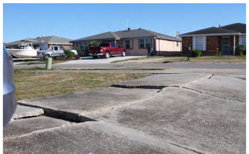
Impact of subsidence on driveways and streets Rain gardens draw water into the ground, which helps with groundwater balance and reducing subsidence, which is the sinking of the ground
