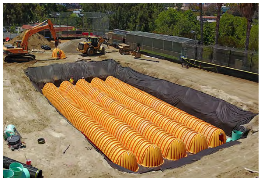
Water storage tanks beneath a field
